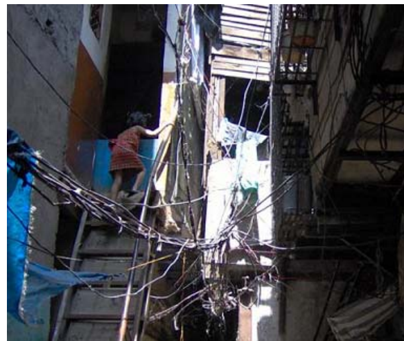
GPOBA project: India Mumbai improved electricity access for slum dwellers; illegal wiring.
